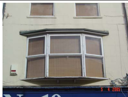
Fig.30 Unsympathetic replacement window
